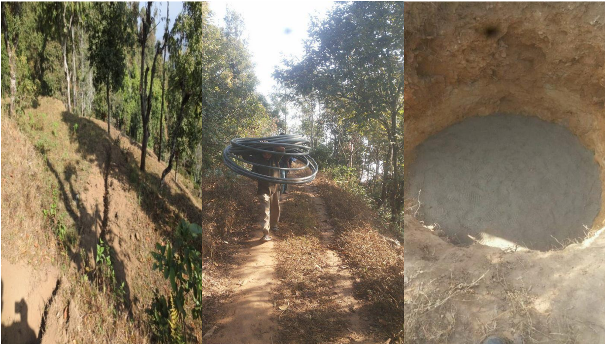
Figure 1: Trench dug for the pipeline, community member carrying water pipe, and pit with sand at the base for the installation of the water tank.
