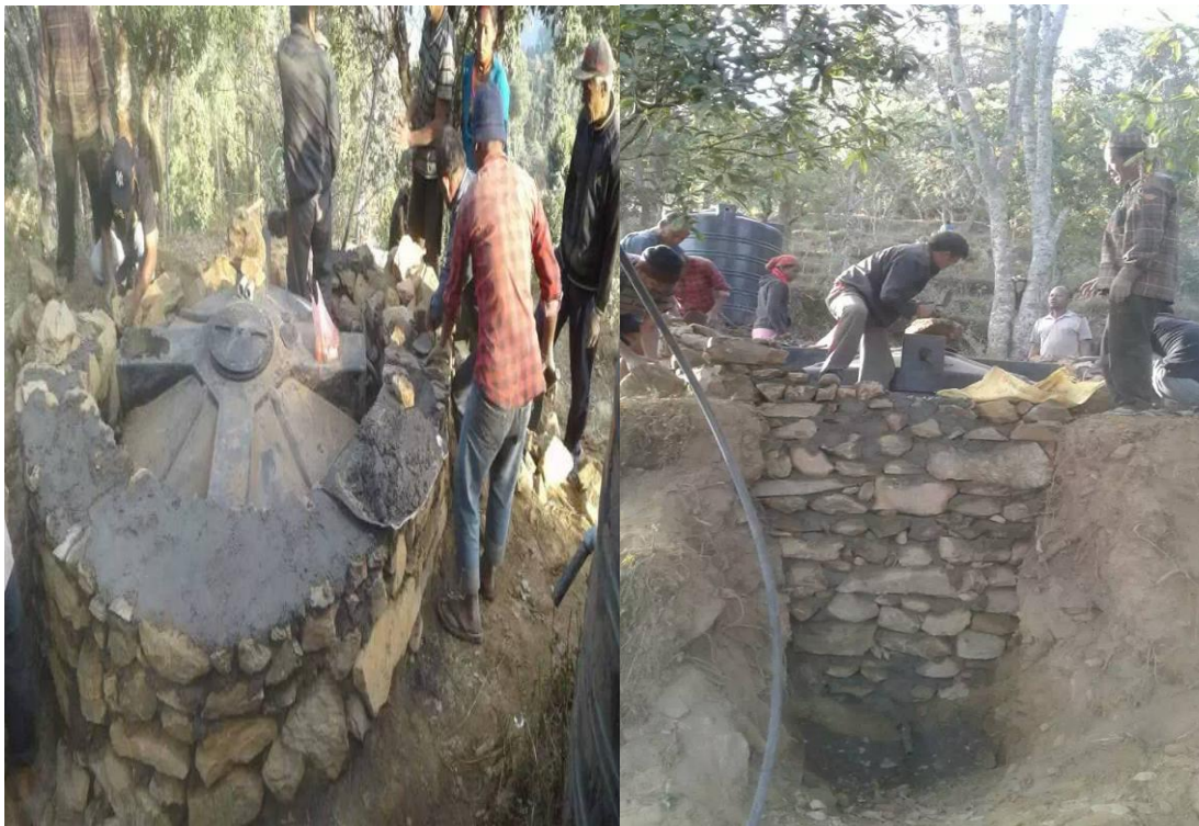
Figure 3: Community members constructing cemented stone-fence for the security of the water tank
