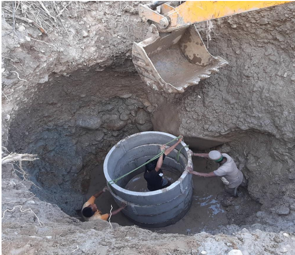
An excavator was used for the site clearance, digging trench, pulling concrete rings for the well construction.
